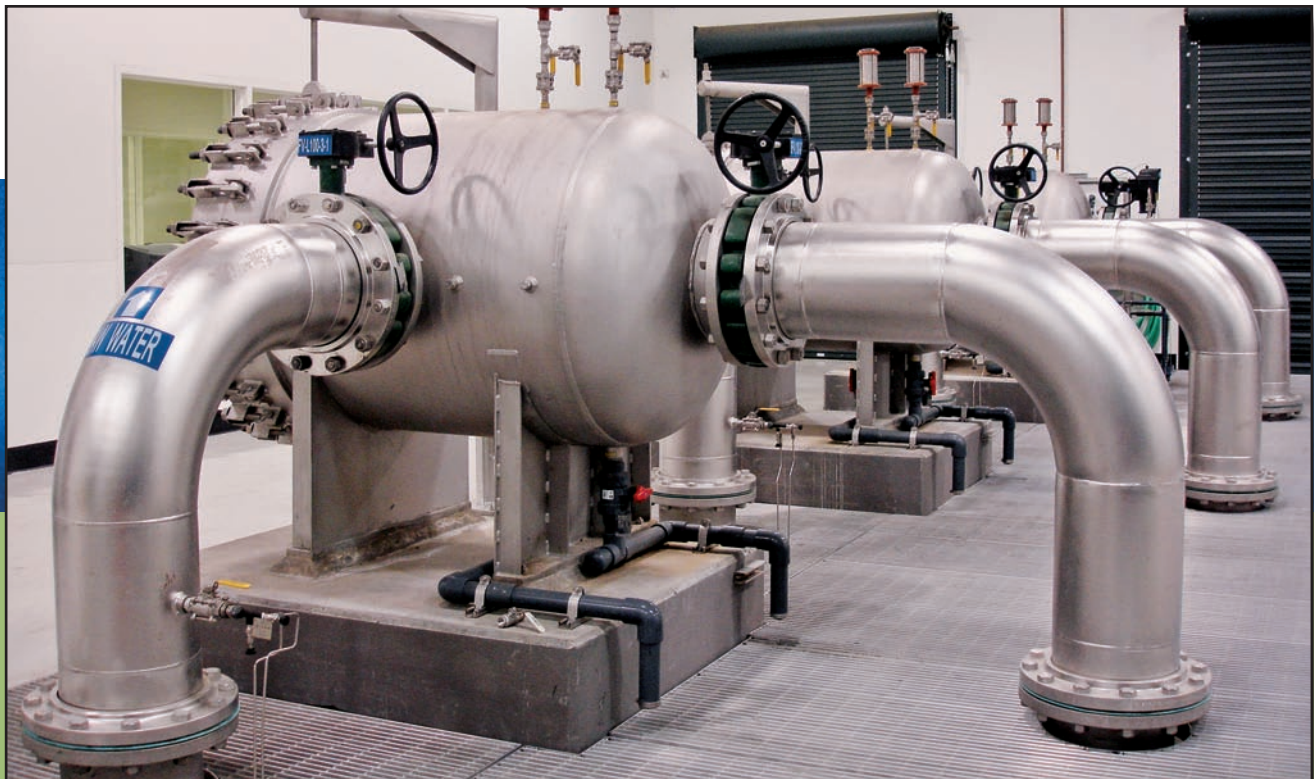
Cartridge filters inside a desalter facility.
