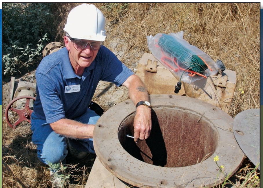
Installing a pressure transducer monitoring device.
