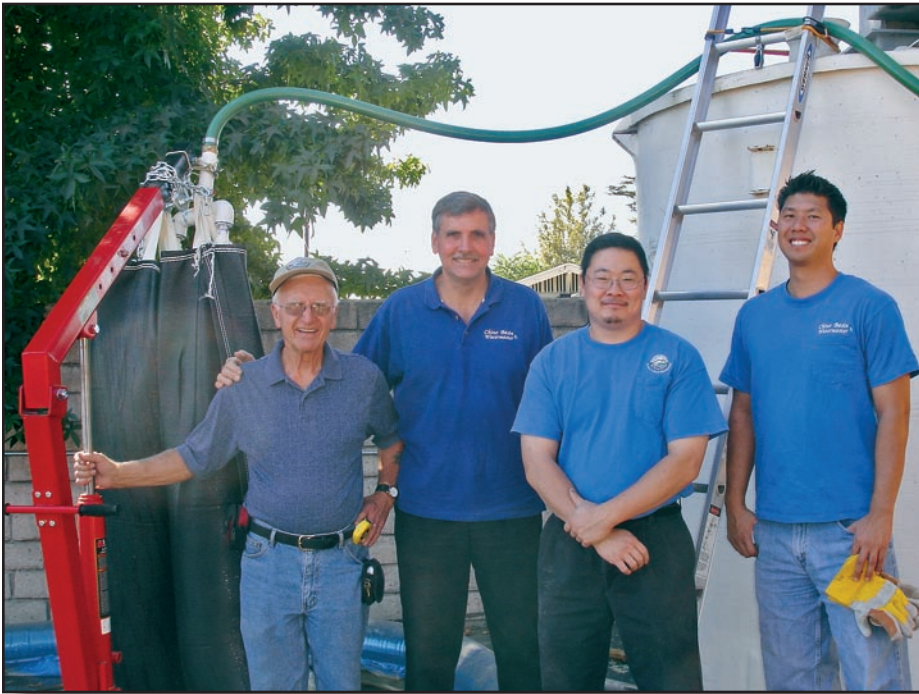
Pilot testing a geo-tube as a dewatering device for recharge basin cleaning.
